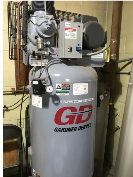
Vertical Reciprocating Compressor
