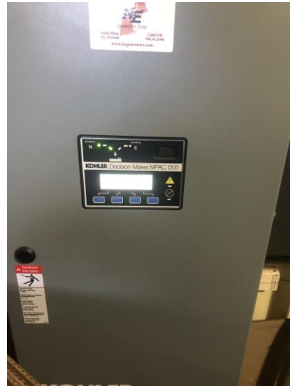
Generator's Automatic Transfer Switch
