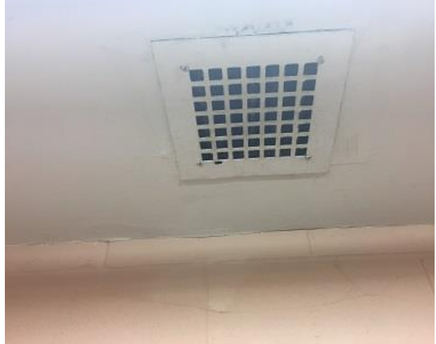
Bathroom Exhaust Grille
