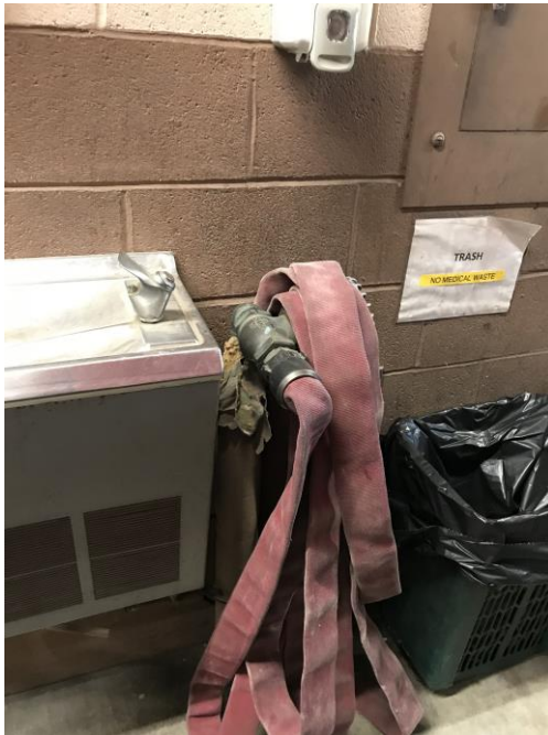
Truck Fill Valve and Drinking Fountain
