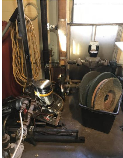
Water Main Entrance
