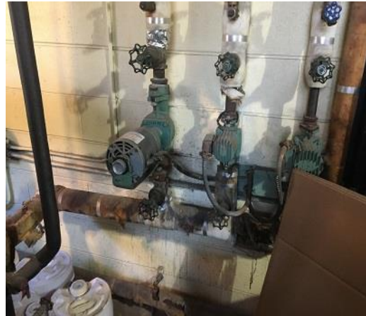
Pump and Piping
