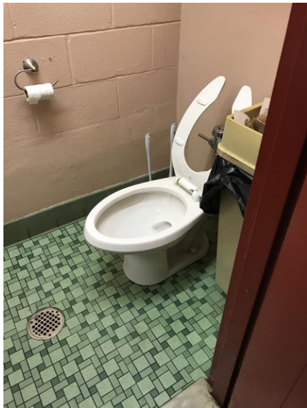
Public Restroom Water Closet
