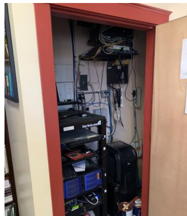
Tel/Data Equipment Rack
