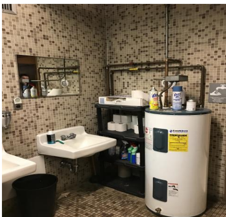
Water Heater & Lavatories
