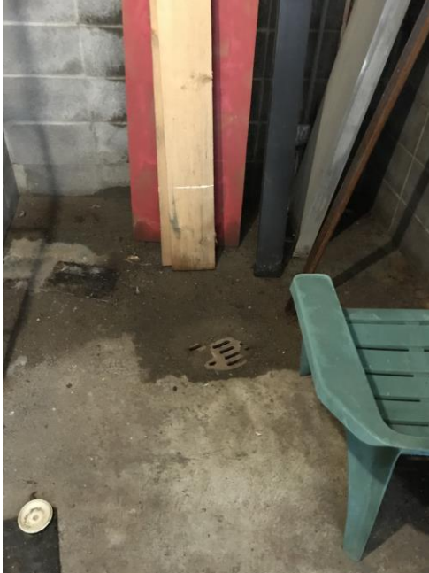
Floor Drain in Hose Tower
