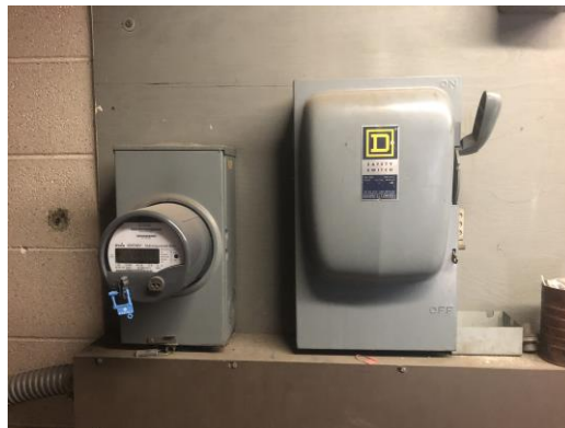
Utility Meter and Main Disconnect
