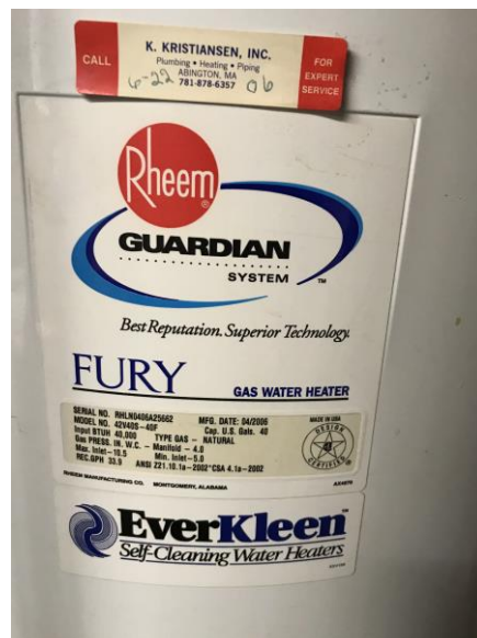
Water Heater Tag
