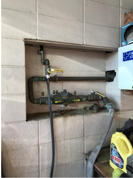
Truck Fill Valve
