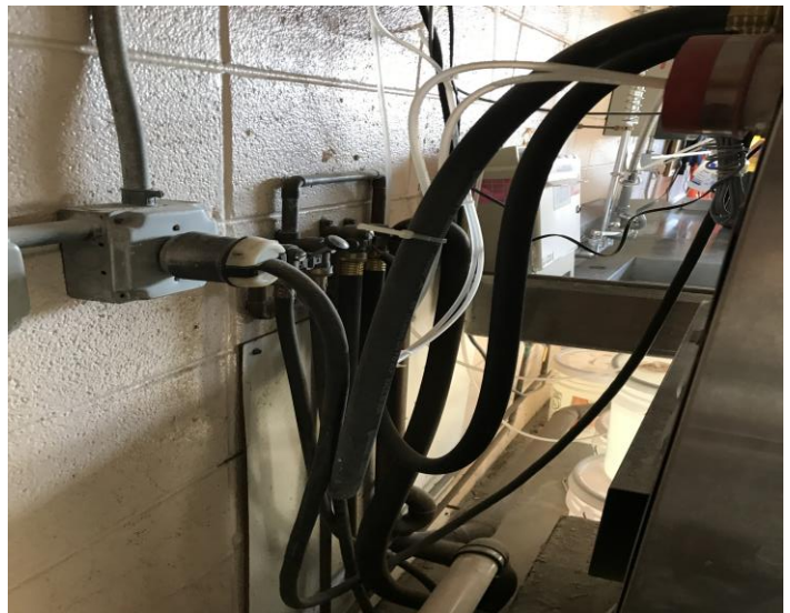
Gear Washer Water Connections
