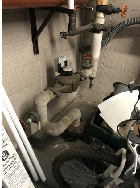
Water Serving Entrance & Water Meter
