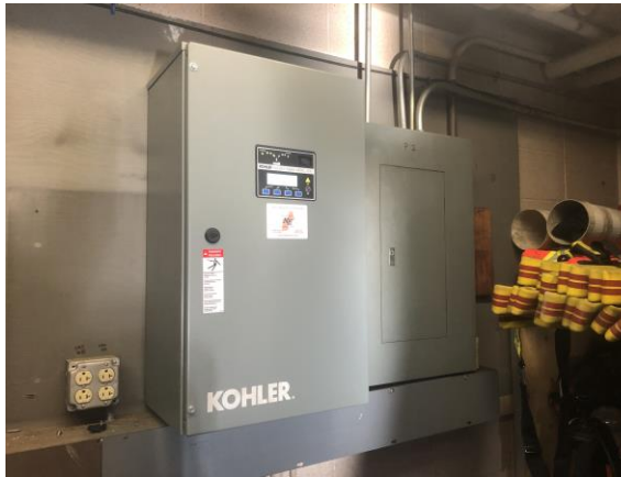
Automatic Transfer Switch
