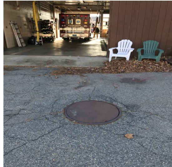
Sand and Grease Trap
